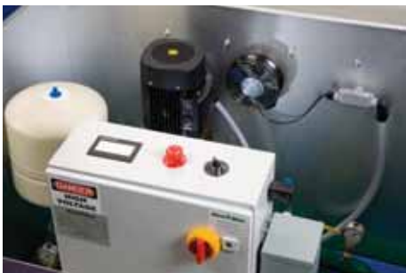
Interior of Low Profile Pump Station (LP)
