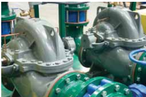
Water Feature Pump Station
