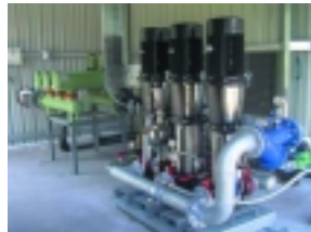
New Rain Bird pump station
