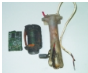
A blown LSP after a lightning strike
