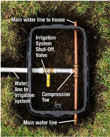
Water meter located outside
