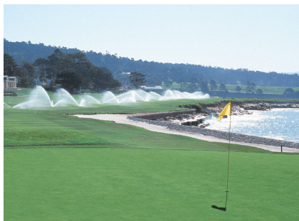
Central control and Rain Bird's IC Rotors communicate instantly with one another. Voltage tests and diagnostics can be run in real time. Make adjustments. Solve problems. Instantly.
