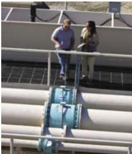
Figure 5. Installation of magnetic meters at the ITRC Pump Testing instrumentation at Cal Poly San Luis Obispo.
